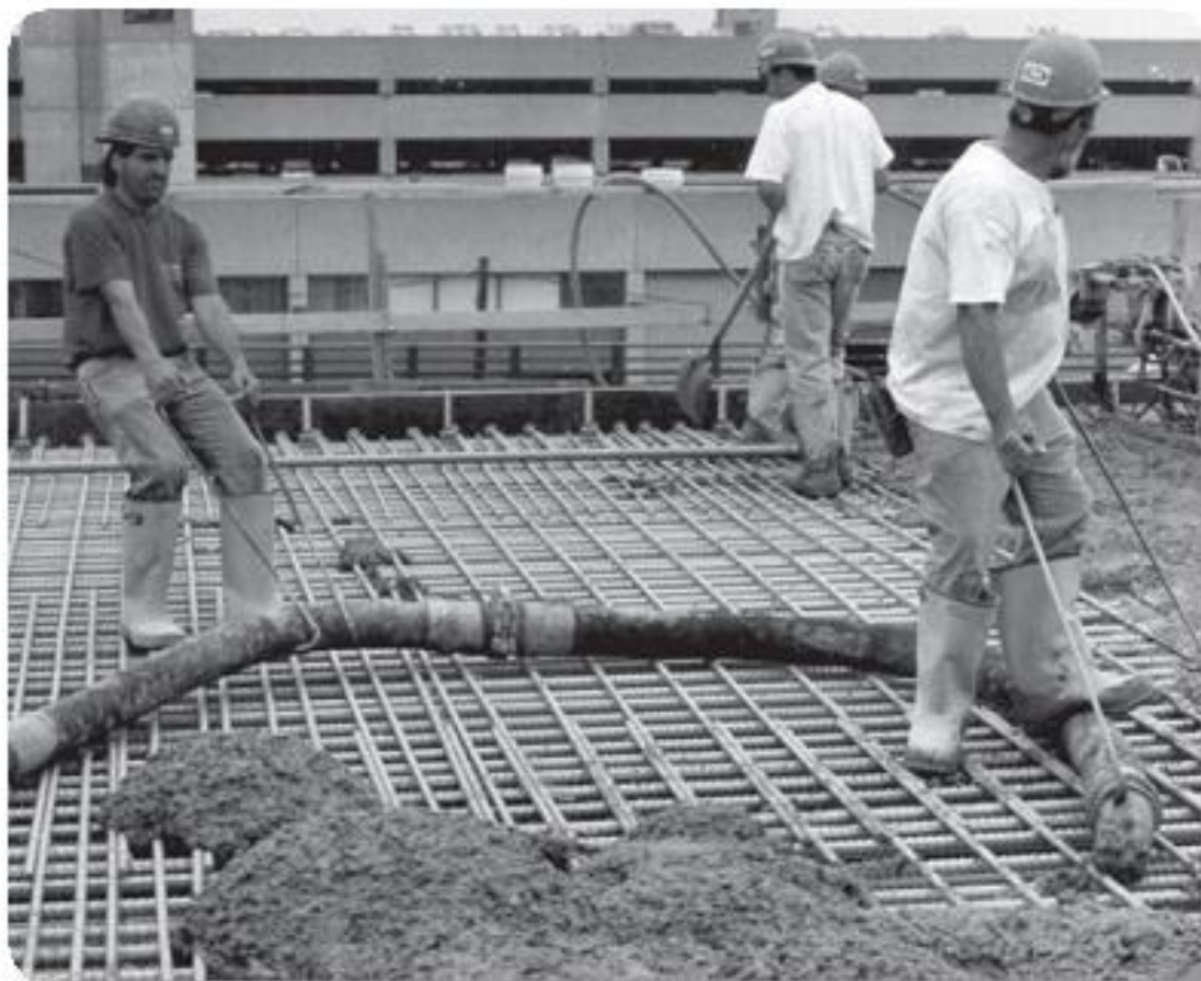
Problem: Pulling concrete hose without skid plate
